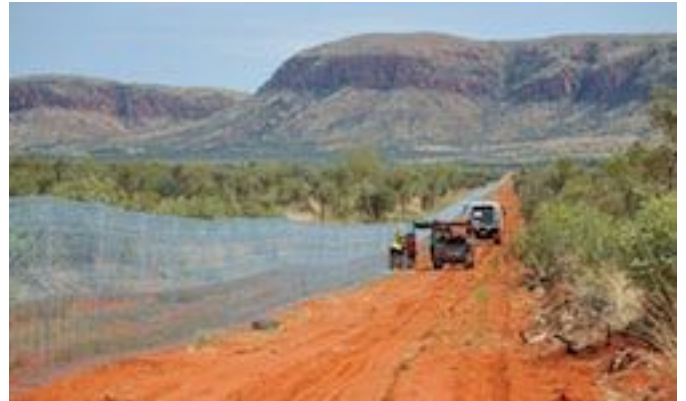
Construction is underway on the 44km fence. Photograph: Wayne Lawler/Australian Wildlife Conservancy
